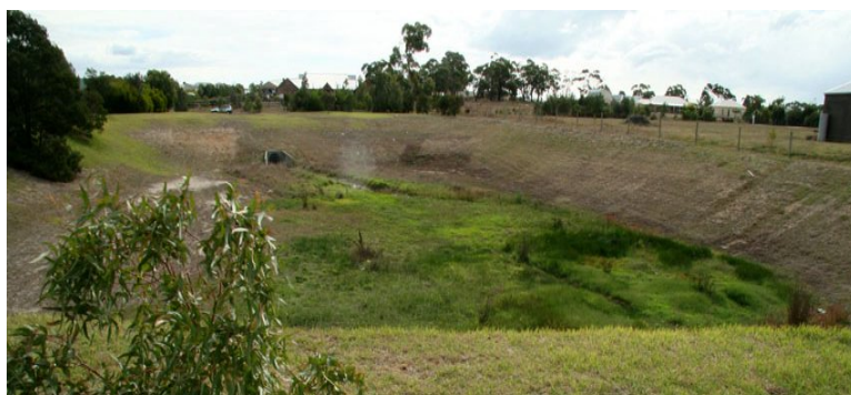
The retarding basin, looking towards Century Drive. The plantings along Balcombe Creek are behind the photographer
