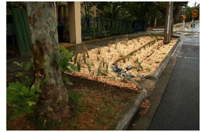
Carroll Crescent, Glen Iris has a series of newly constructed rain gardens, planted with reeds, and mulched with pebbles, and fed by water from the gutter.
