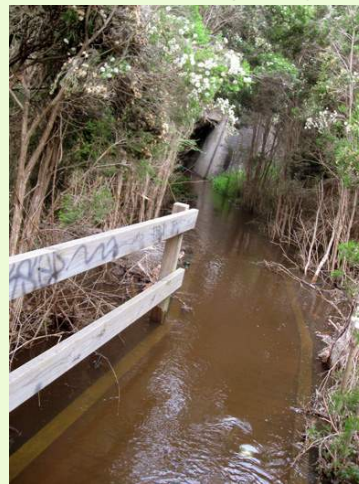
The inundated boardwalk just downstream from the Uralla Rd bridge.
